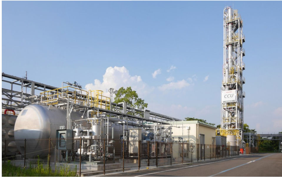
CO 2 Capture System at the Duiven WTE Facility (Netherlands). SOURCE: The Global CCS Institute
